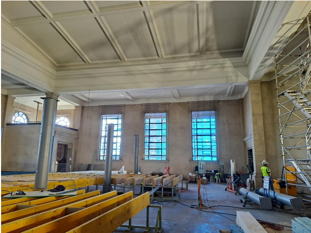
Figure 7: Looking north within auditorium, location of proposed lift between centre and right window
