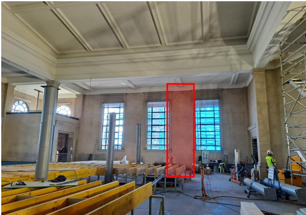
Figure 12: Northern wall of auditorium with the approximate location of the proposed lift marked
